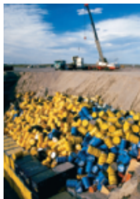
Figure 20 A crane lowers drums of radioactive waste into a landfill in Hanford, Washington.
